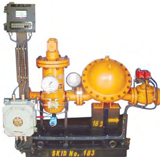
MSA meter skid with Toptech SMP controller
